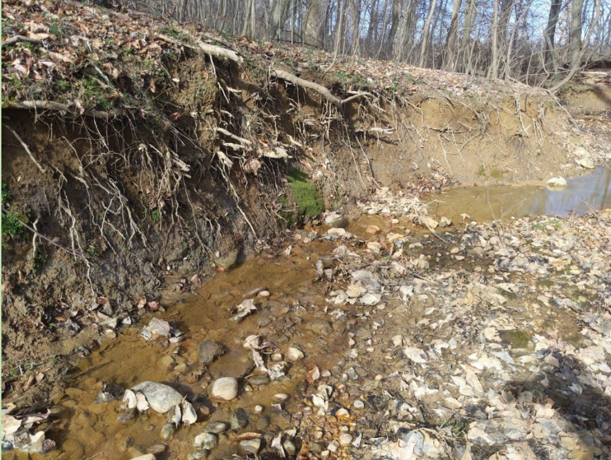
Typical laterally eroding bank
