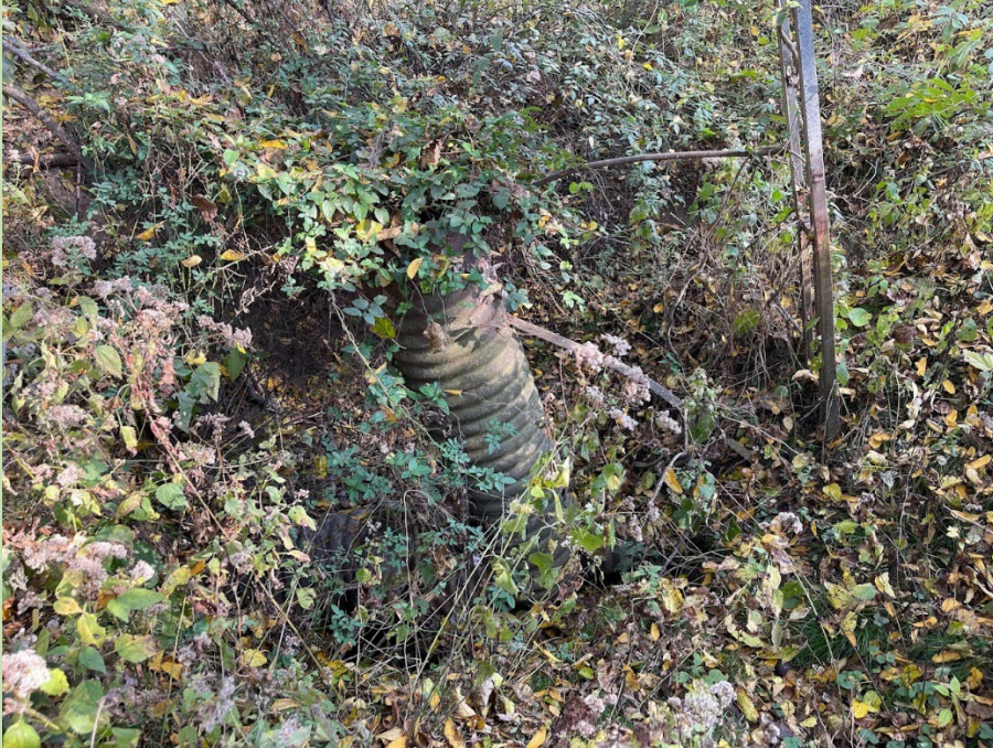
Site B- failed primary control structure in-stream at failing historical berm installed in 60s or 70s.
