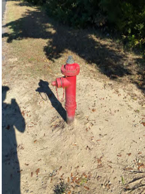
Photo 6. Phase 3 - Hydrant Line along Proposed Access Road
